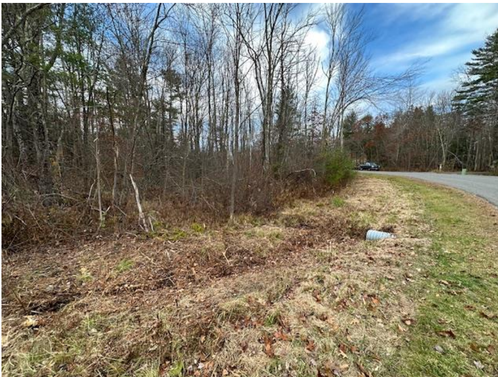
Photo 2: The subject wetlands and lot drain to this culvert point which conveys flows under Sherbrook Drive.
